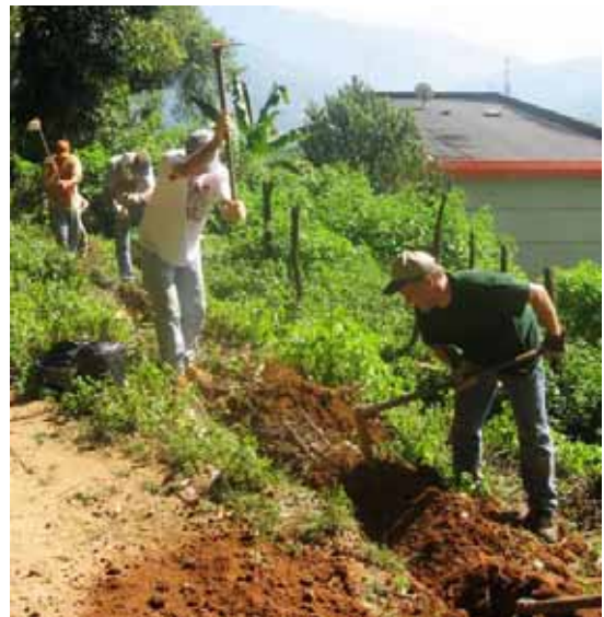
Team members from Texas and Church of All Nations in Hong Kong dug trenches and laid piping for a water system on a recent service trip in China
