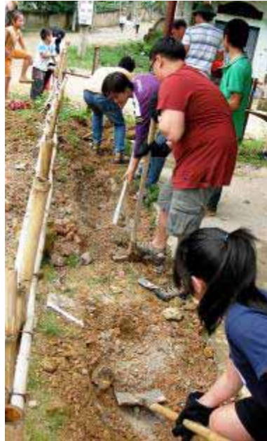
Team members from Seoul Foreign School work to dig a foundation for a boundary wall on a recent trip to Vietnam
