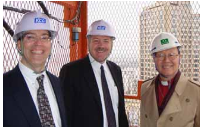
Carl Hanson (LCMS WM Area Facilitator, East Asia), John Mehl (LCMS WM Regional Director, Asia), and Dr. Um (LCK President) riding 24 stories above Seoul in a construction elevator on the outside of the Lutheran Church in Korea's new building – which is planned to generate additional funding for expanded mission and ministry. The building is scheduled to be completed in July with a formal dedication ceremony planned to coincide with the annual convention of the LCK in the first week of October.
